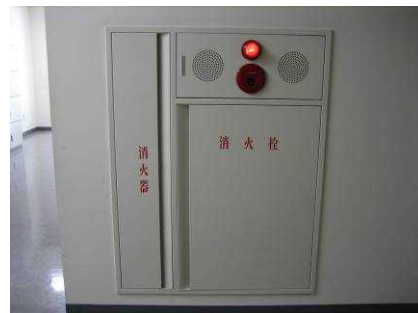
Fire alarm (top) and hydrant (bottom)
